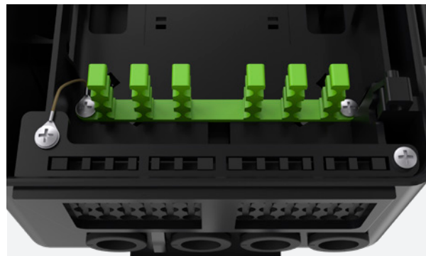
Cable Tie Points
